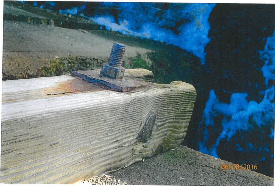
Photo 15: West side, 7th post from the south has missing anchorage on the bottom.
