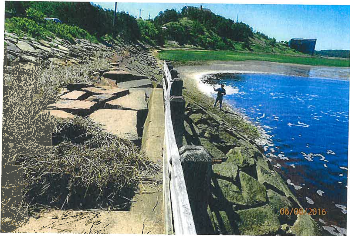
Photo 13: Typical deflection of rail following settlement of wingwalls on flume extension.
