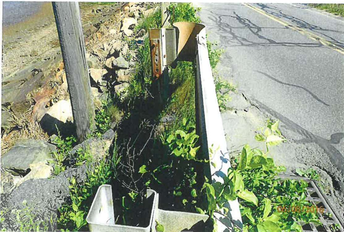
Photo 22: NW gloved end and first section of rail is cantilevered (not connected at end).
