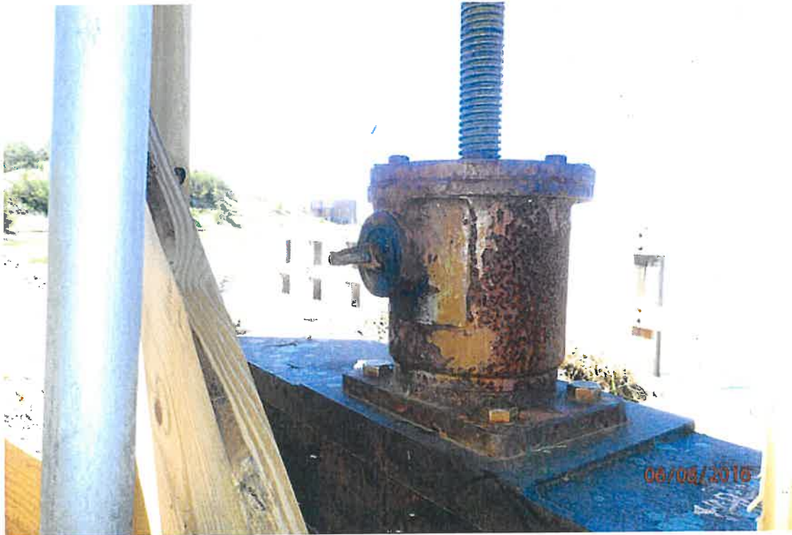
Photo 23: SW gate control mechanism appears to be non-functional.
