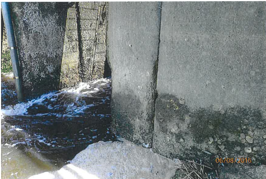
Photo 6: Spalls on downstream south barrel south wall.
