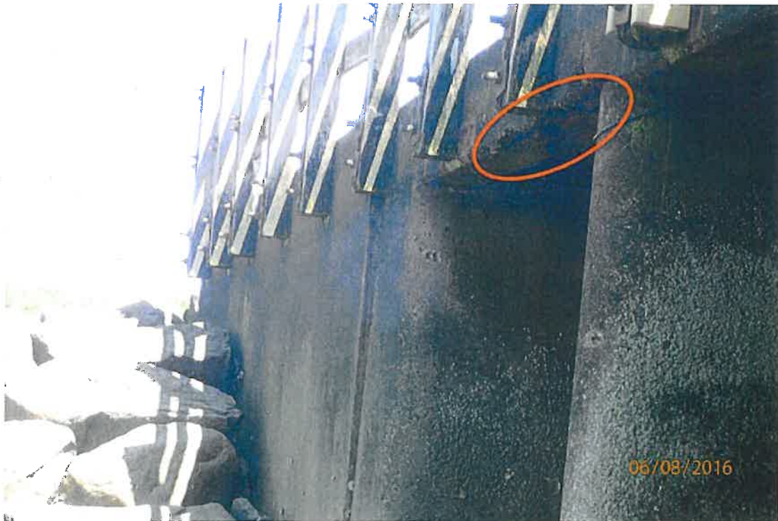
Photo 4: Headwall of downstream flume extension has spall.
