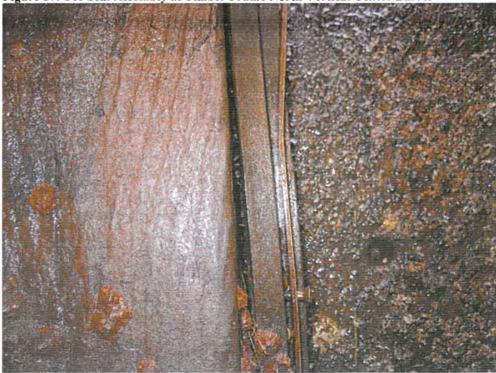
Figure 18: Tee Seal Assembly (inadequate seating and fastening to substrate)
