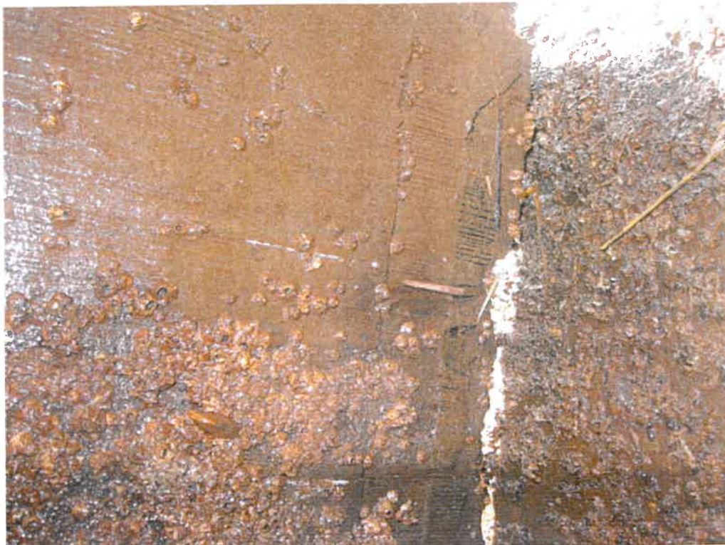
Figure 13: Deteriorated Tide Gate at Seating Surface North Edge Center Barrel
