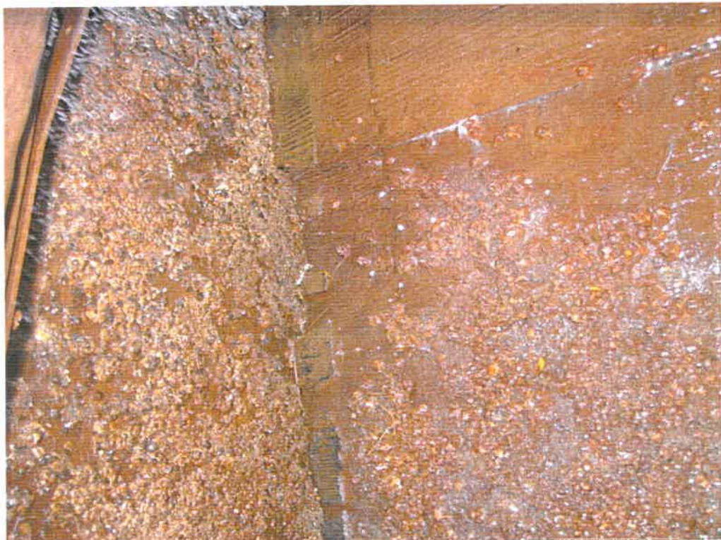
Figure 12: Deteriorated Tide Gate at Seating Surface South Edge Center Barrel
