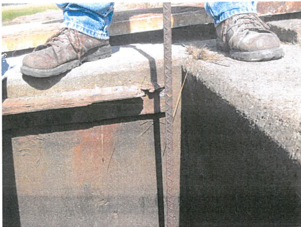
Figure 23: Advanced Structural Distress Grating Support
