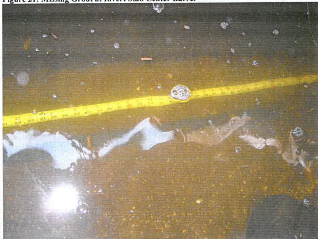
Figure 22: Missing Grout at Invert Slab Center Barrel
