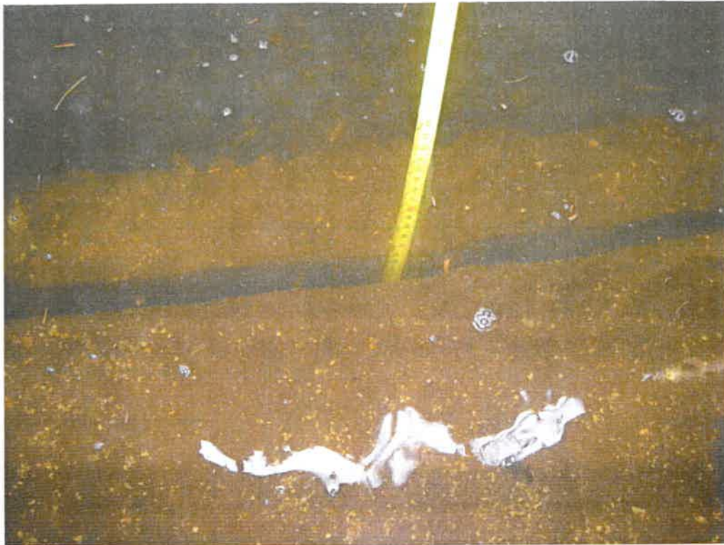
Figure 21: Missing Grout at Invert Slab Center Barrel
