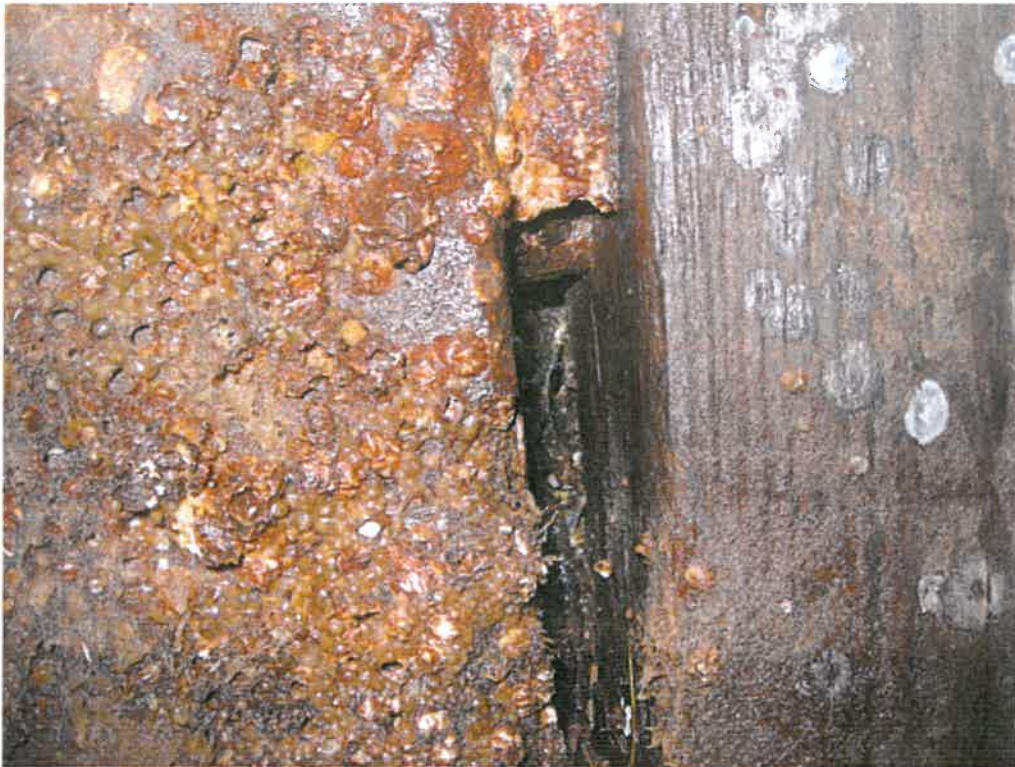
Figure 19: Missing Grout North Barrel South Vertical
