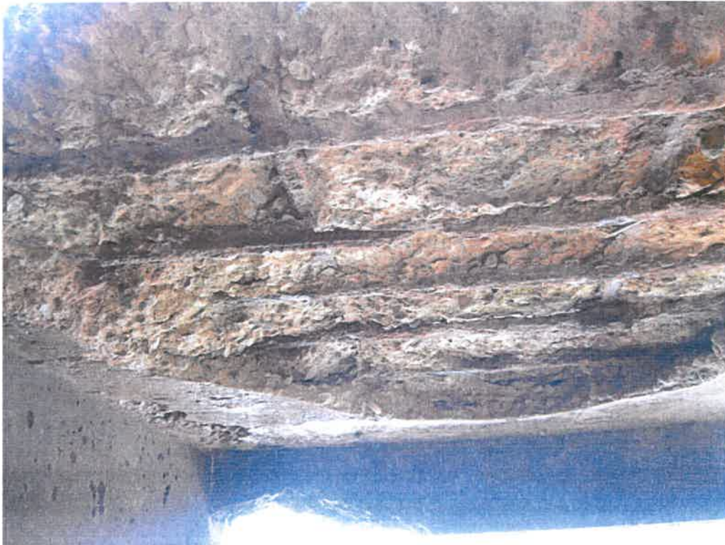
Figure 25: Advanced Deterioration of Reinforcement at Deck Slab Spall over Flume
