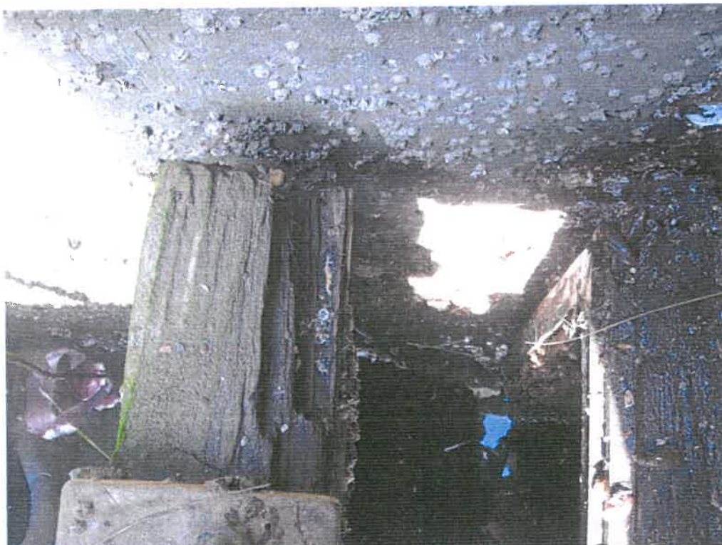
Figure 14: Deteriorated Tide Gate at Timber Frame Header
