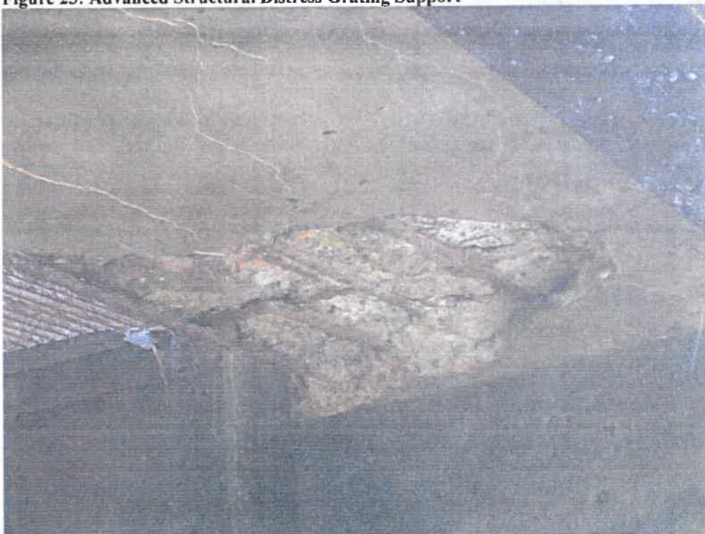
Figure 24: Deck Slab Spall over North Barrel Flume
