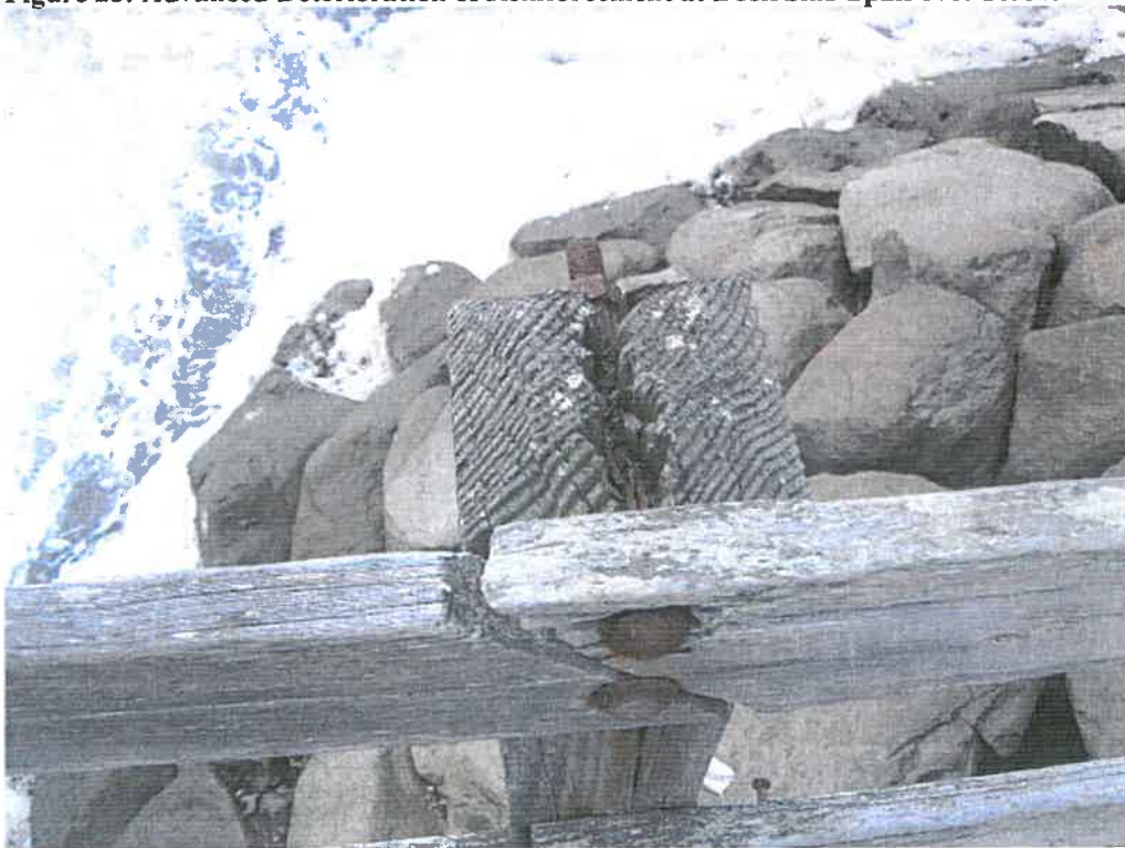
Figure 26: Typical Safety Railing and Post
