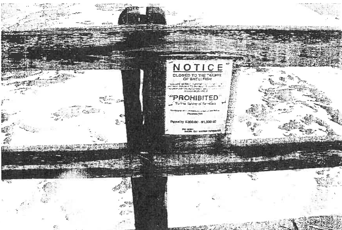
Photo 8: All railing posts are split (this one full hieght) most likely to pack rust of mounting bolts
