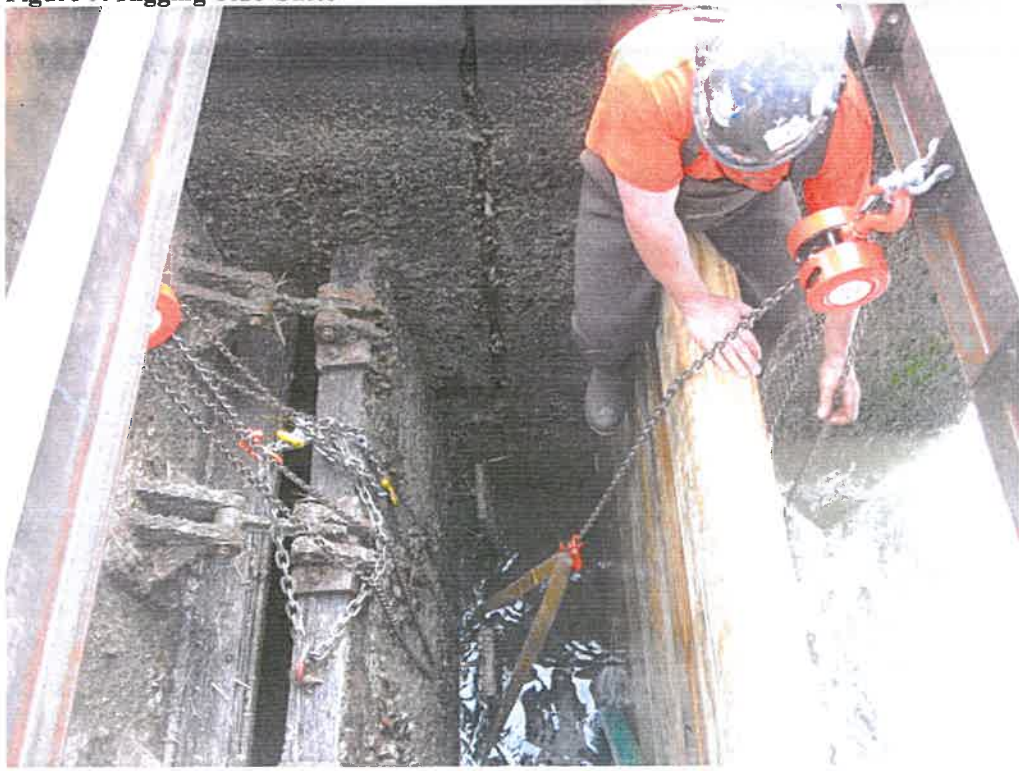
Figure 10: Actuating Tide Gates
