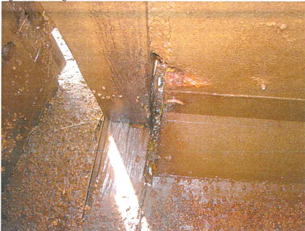
Figure 20: Missing Grout Center Cell at Roof Slab North (note: Spall at Roof Slab)
